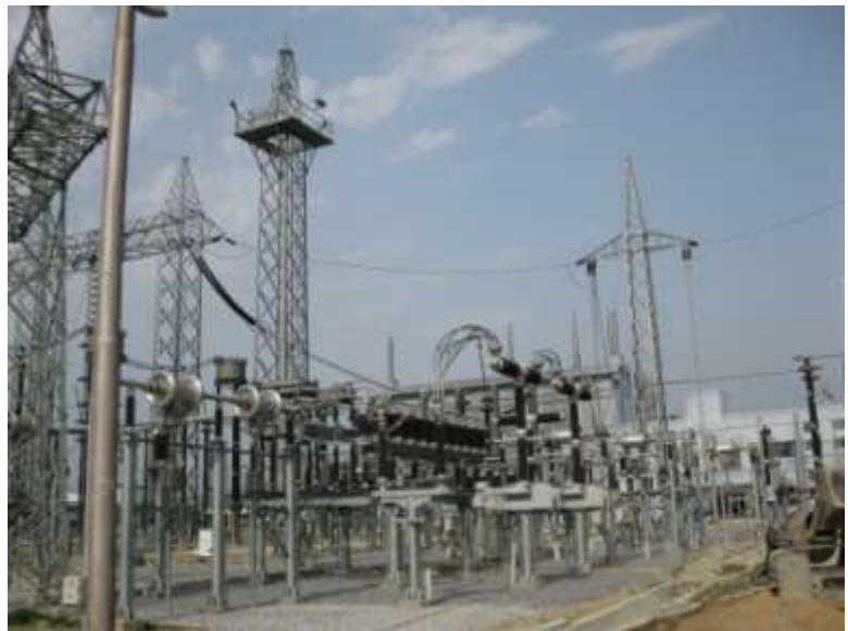
Picture 4: Converter substation
